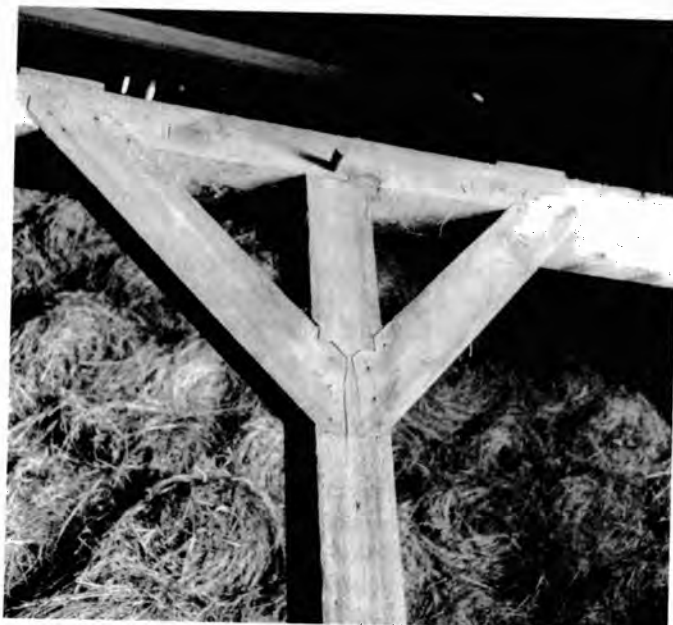
Detail of barn construction. Note the fitting and lack of nails. This was typical of the late 19 th century architecture in the street villages of the West Reserve. Photo credit: Harold Funk
